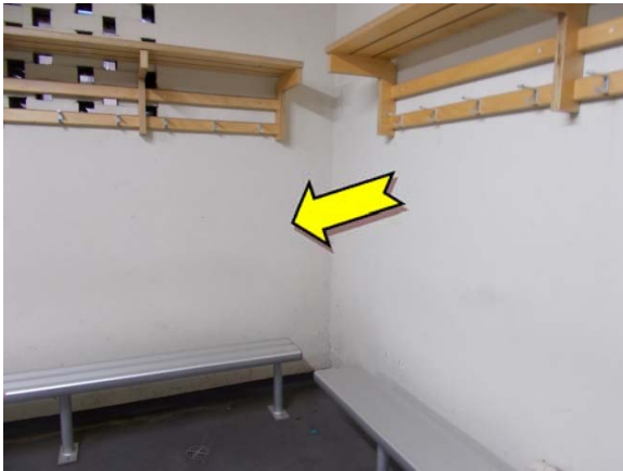
Photo 9. Interior, ground level, dressing sheds, throughout, walls – suspected lead-containing cream upper paint systems.
