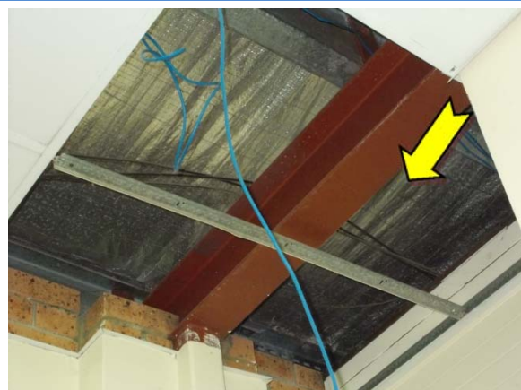
Photo 6. Interior, level one, throughout, roof space, insulation – suspected SMF sarking insulation material.
