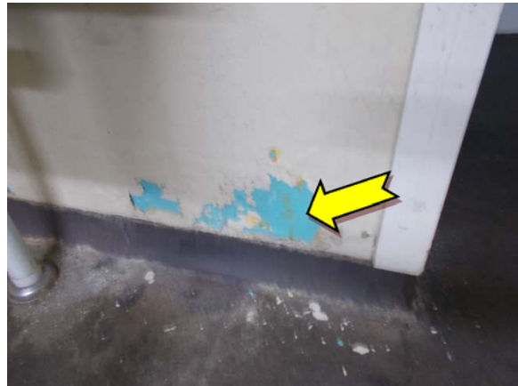
Photo 10. Interior, ground level, home dressing shed, walls – suspected lead-containing light blue lower paint systems.
