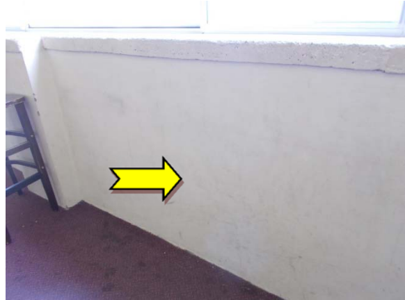
Photo 8. Interior, level one, throughout, walls – suspected lead-containing beige upper paint systems.
