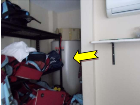
Photo 7. Interior, ground level, laundry room, hot water heater – suspected internal SMF insulation material.
